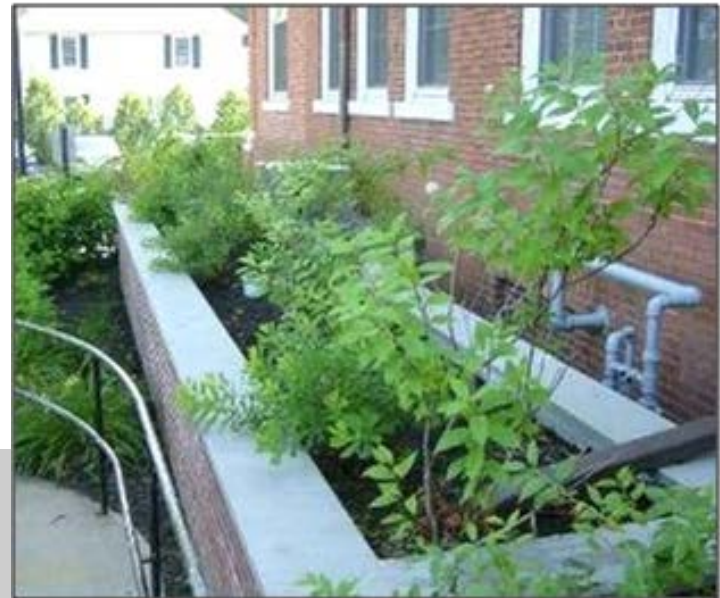
Infiltrating planter box designed to capture and treat rooftop runoff (Plymouth, MA).
