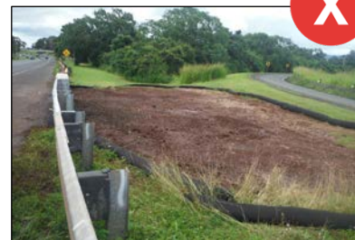
Install non-vegetative erosion controls, to the extent necessary, to provide cover to areas where vegetation is becoming established.
