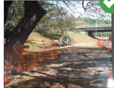
Steel plates were installed under the tree drip line to protect the root system after consultation with a licensed arborist.
