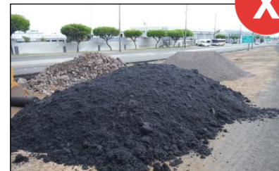
Cold patch spoil piles or waste asphalt piles must be placed on and covered with impervious material, as well as have full perimeter control around the base of the stockpile.
