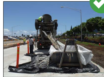
Concrete washout area must be lined with an impermeable material. Secondary containment under washout catches any leaks or splashes from the washout area.
