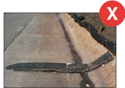
Check dams that get flattened must be repaired/replaced.
