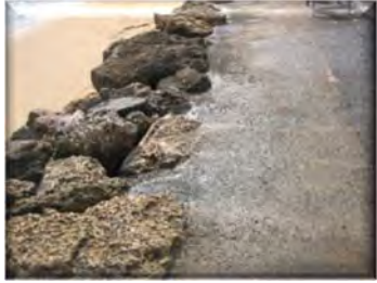
Tidal sand on the road.
