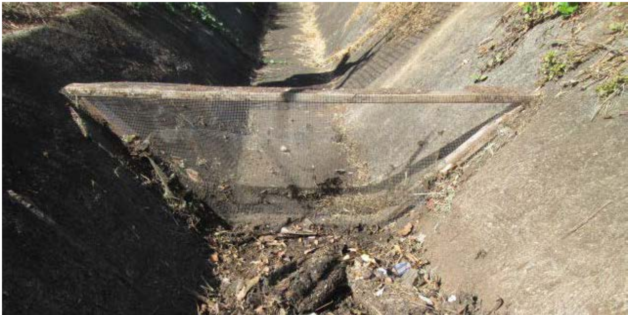
Figure 4. Trash trap located at Site #3.
