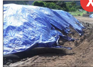
Damaged covers and gaps in perimeter protection increase the chance of water or wind erosion from the contents of the stockpile.
