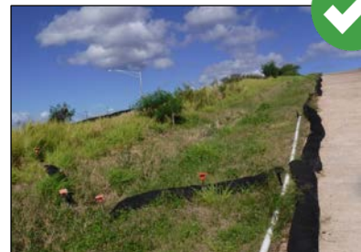
Follow manufacturer’s specifications on proper use for fiber rolls used as velocity dissipation devices on steep slopes.
