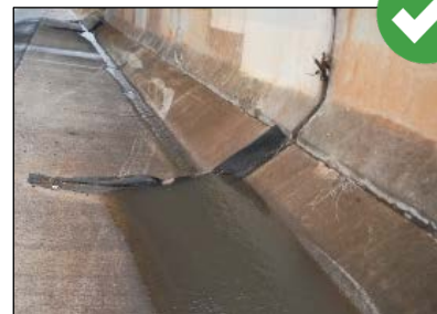
The center of the check dam must be lower than the ends to prevent water from running around the ends and causing additional erosion.
