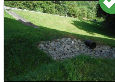
High flow velocities at the pipe outlet require the implementation of velocity dissipation devices to prevent downstream erosion.
