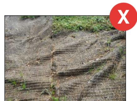
Matting must maintain direct contact with soil to prevent rills, gullies, and undermining.
