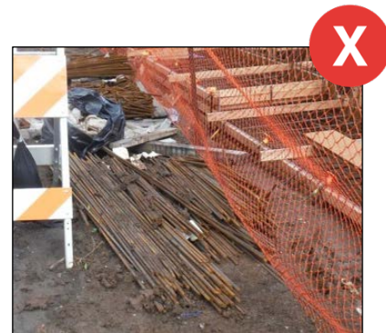
Galvanized metal and rebar must be racked off the ground and covered with impermeable material.
