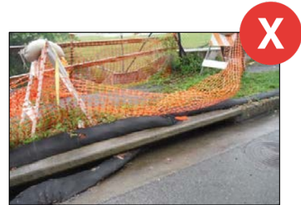
If inlet protection BMPs are falling into the inlet, they must be pulled out and repositioned, per manufacturer's specifications.
