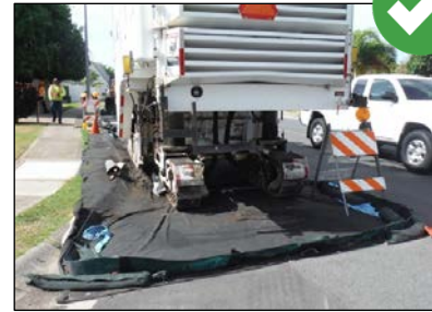
Idle paving equipment must be stored drip protection to contain leaks and spills.
