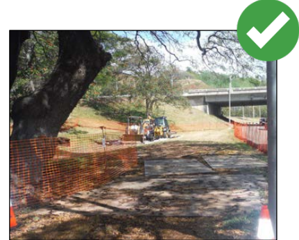
Steel plates were installed under the tree drip line to protect the root system after consultation with a licensed arborist.
