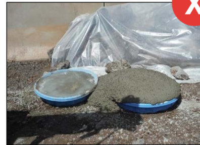
Concrete washouts must be changed or not used after reaching 75% capacity or 4-inch freeboard, whichever is more stringent. Hardened concrete should be removed frequently to avoid overcapacity of washout area.
