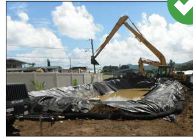
Construct sediment trap prior to engaging in clearing, grubbing, or grading activities.
