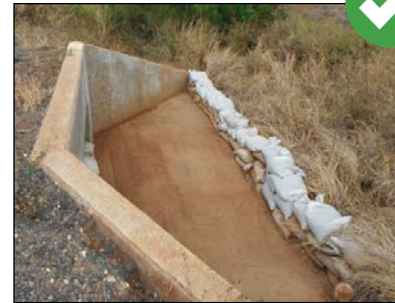
Sandbags may be stacked in a brick wall-like formation if additional reinforcement is used.
