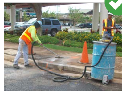
Properly vacuuming saw cut and boring slurry prevents the slurry from entering storm drain systems and adjacent waterbodies.
