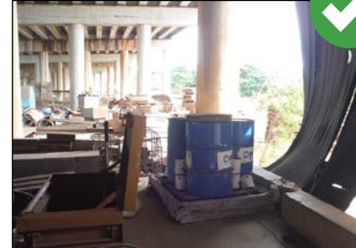
Metal containers must be covered by an impermeable material or under a covered facility to prevent contact with rainwater, which can cause rusting and potential leaks.
