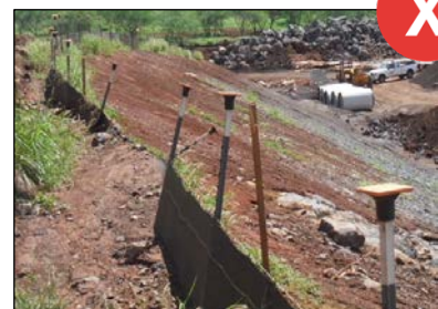
Avoid using silt fences on slopes. However, if silt fence is placed on a slope, the fence post may need additional embedment.
