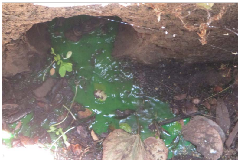
A dye test verifies the connectivity of a private drainage structure to the DOT-HWYS MS4.
