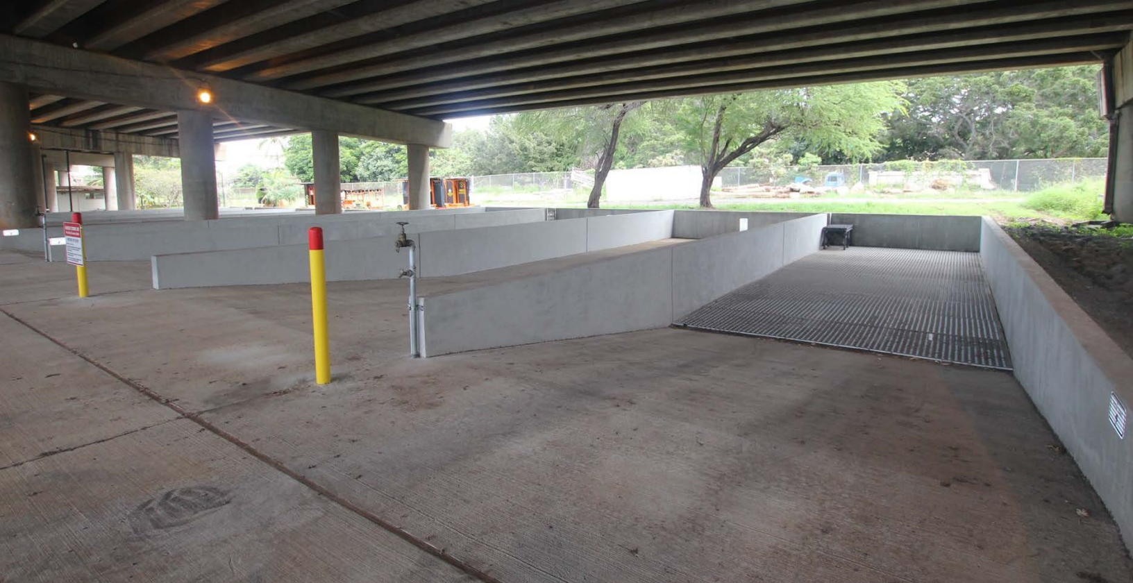
A Dewatering Facility is located at Pearl City Baseyard, Pearl City, Hawaii.
