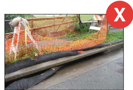
If inlet protection BMPs are falling into the inlet, they must be pulled out and repositioned, per manufacturer's specifications.
