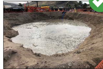
Dewatering pits may be pumped with water from dewatering operations so construction activity may be accomplished.
