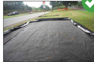
Store vehicles and equipment on a layer of geotextile filter fabric on top of 10 mil plastic sheeting when not being used.
