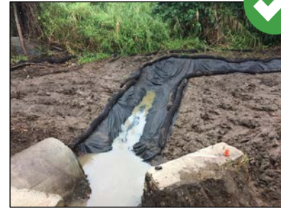
Swales and ditches can be used to intercept, divert, and convey surface run-on to a stabilized area or other sediment trapping device.
