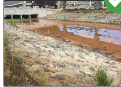
Inlets, outlets, and slopes of sediment basins must be stabilized with rock or vegetation to minimize erosion.
