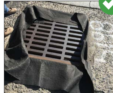
Properly installed geotextile filter fabric is placed underneath the grate and extends 6 inches past the grate on all sides.
