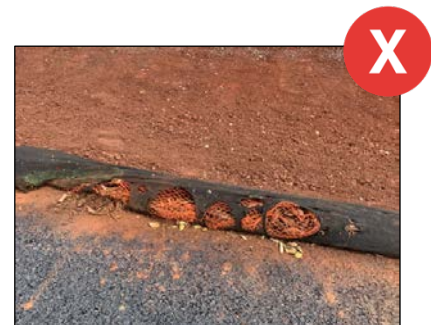
Repair/replace split, torn, or slumping compost filter socks to preserve filtration capabilities.
