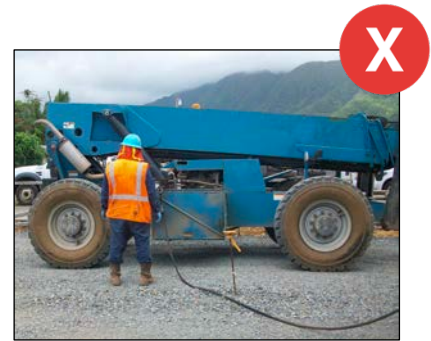
There must be drip protection under vehicles and equipment that are being refueled on-site.
