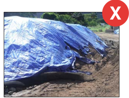
Damaged covers and gaps in perimeter protection increase the chance of water or wind erosion from the contents of the stockpile.
