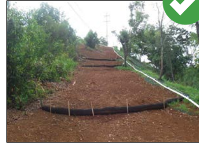
Compost filter berms must be staked into the slope to secure them into the ground.
