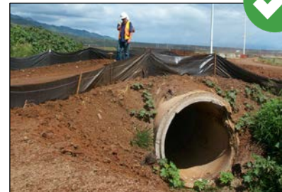
Culvert crossings must be properly sized to minimize erosion and maintain stream flow.
