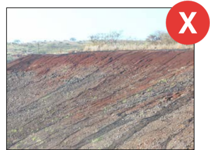
Additional mulch may be needed if erosion of hydroseeded area has occurred.
