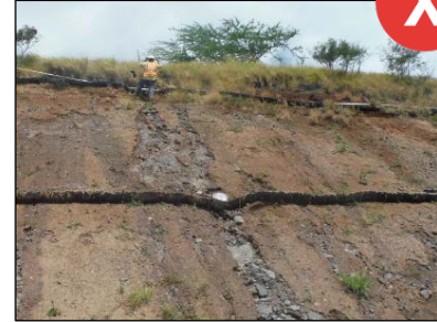
Compost filter berms that do not maintain direct contact with soil allows erosion and undermining to occur.
