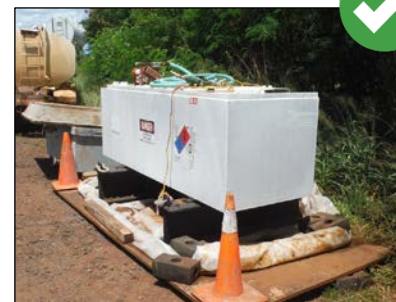
Protect on-site fueling areas with berms and dikes to prevent run-on, runoff, and to contain spills.
