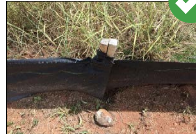
Properly installed silt fences are overlapped between adjoining segments or are overlapped, wrapped, and rolled.
